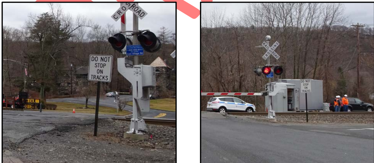
Figure 6 - Do Not Stop on Tracks sign
